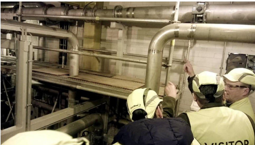
Image 1: The OxTube DN200 is running in a paper mill waste water treating plant by UPM.
