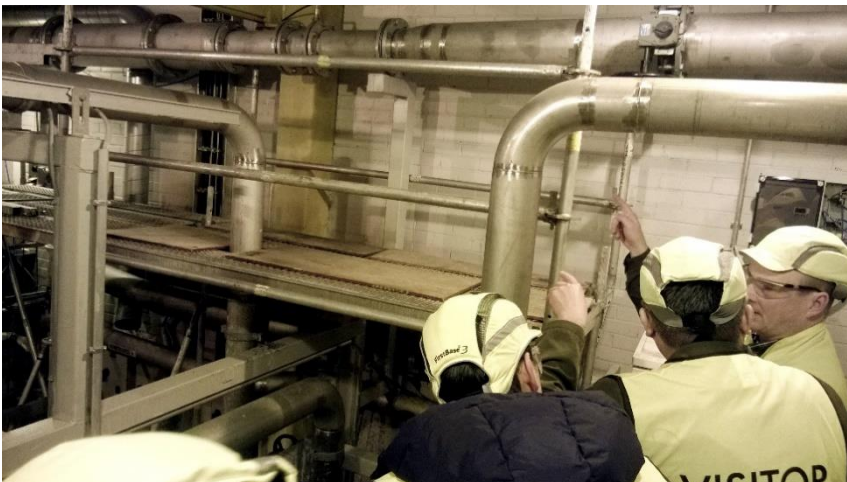
Image 1: The OxTube DN200 is running in a paper mill waste water treating plant by UPM.
